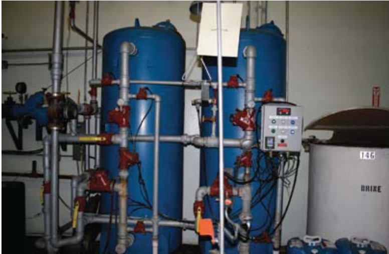
A view of water softening equipment
