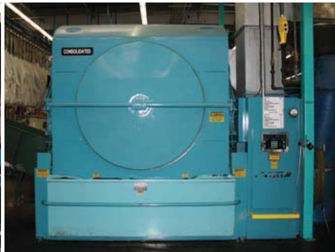
A CLM dryer in the wash aisle
