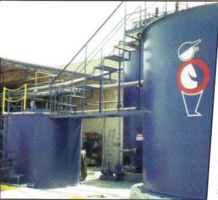
The Wastewater Treatment tanks at Fresno.
