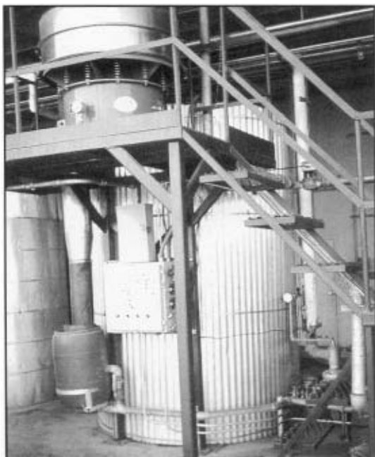
The Fresno Plant hot water reuse system has an elevated shaker on top of the heated tank which holds the water ready for reuse.
