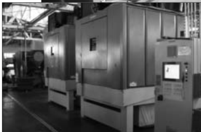
The Irvine Plant dryers
