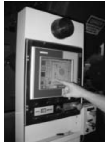
Microprocessor - Each washer has its own microprocessor to control washer functions and communication with the overhead rail system.
