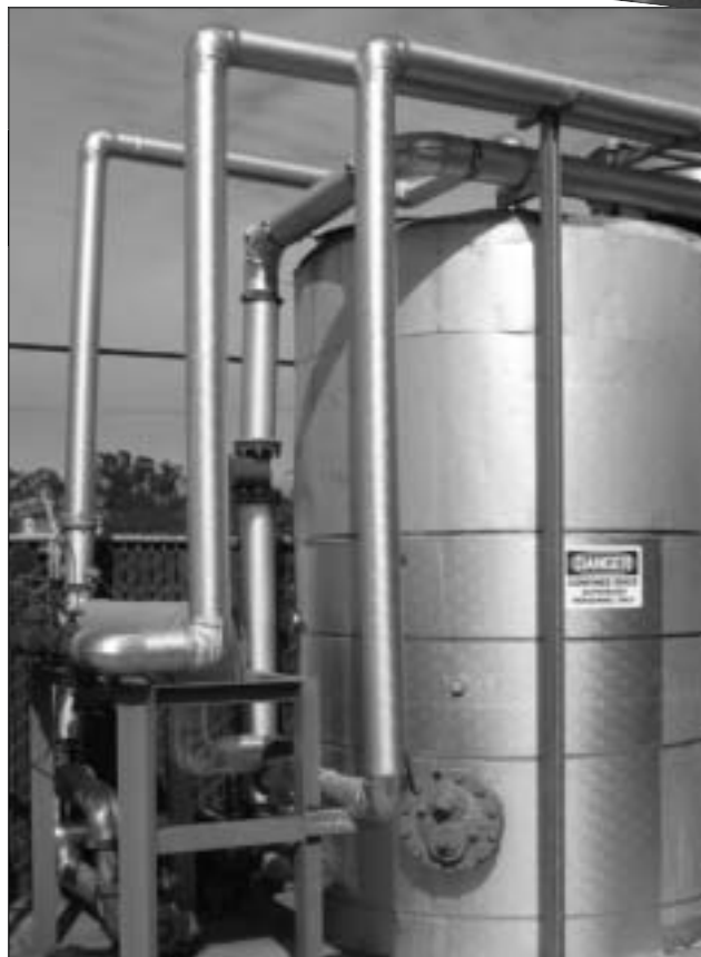
The Irvine Industrial Plant has a state-of-the-art water reuse system. This system has an external side steam coil. This heating device provides steam from a boiler that maintains a high temperature in the reuse tank.
