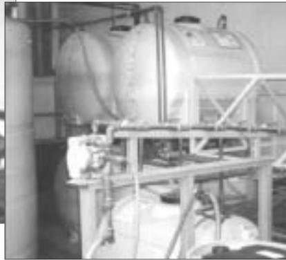
The outside tanks connected to the Injection System.
