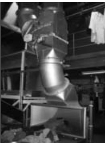
Dryer Vacuum System – Vacuum system carries garments to the dryers which are on a mezzanine above the washers.
