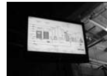
Spindle – The Spindle system tracks utilities and plant operation on this central display (refer to page 18 to learn more about Spindle Technologies).
