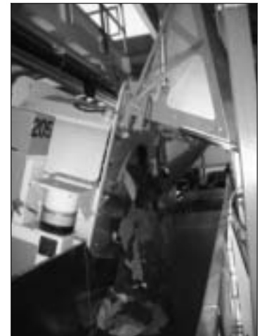
Washer Unloading – Washer automatically unloads onto a conveyor which is used to transport garments to dryers.
