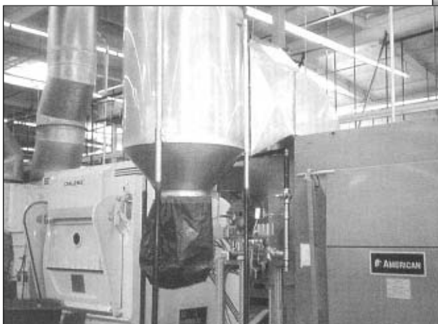
The Vista Plant lint trap connected on the dryer.
